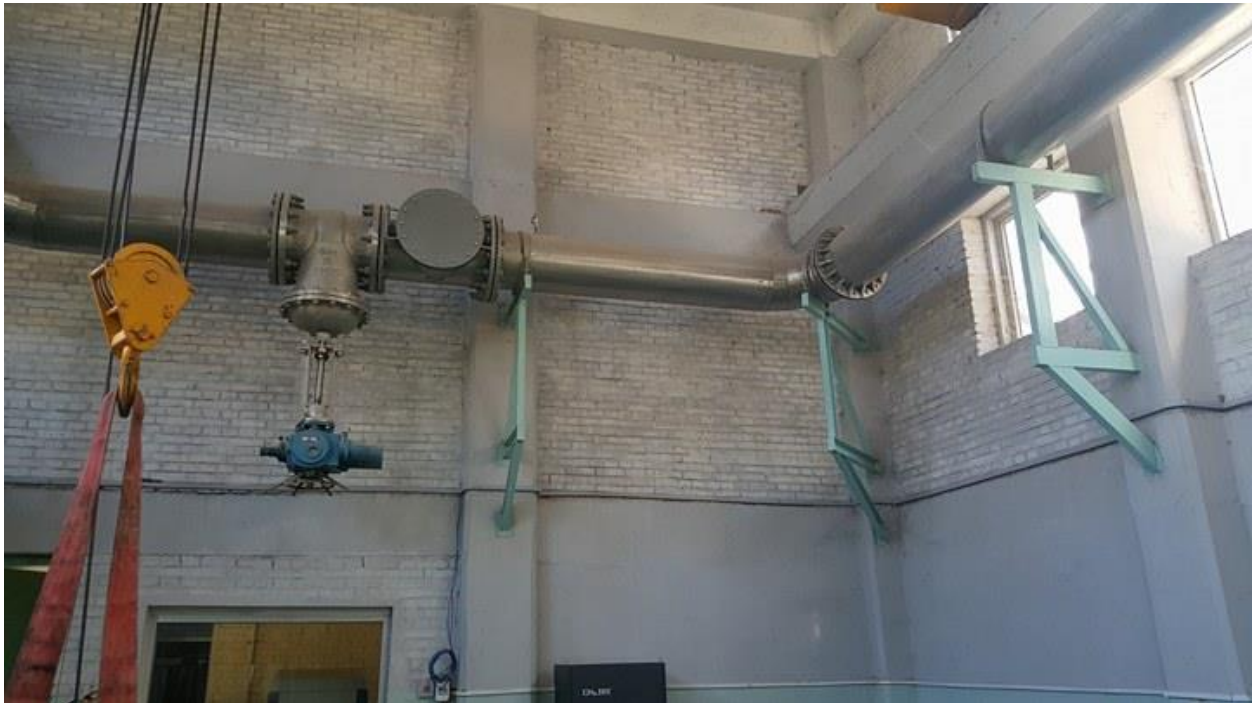
Picture 1: Current position of the valve and the connection
