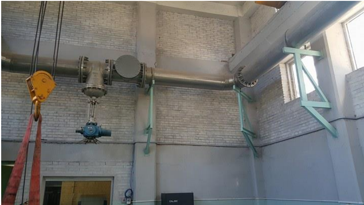
Picture 1: Current position of the valve and the connection
